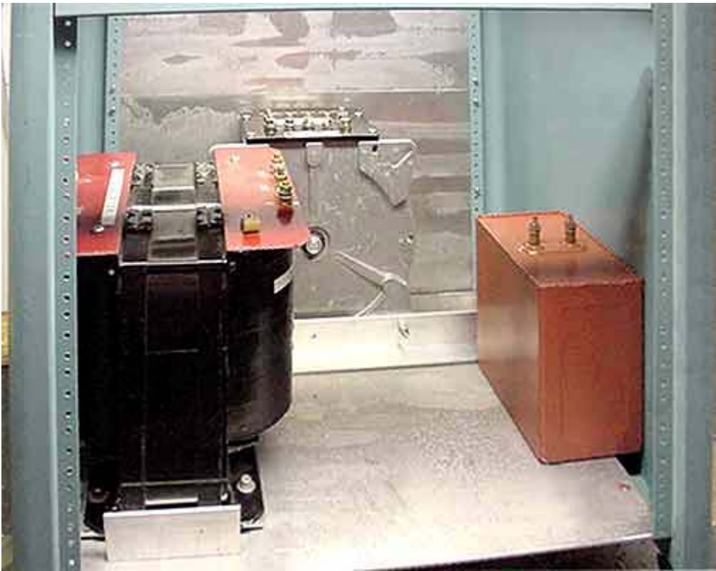
Power supply cabinet at beginning of construction. This shows (1) the plate transformer, with a 240V primary and 3500V, 2A CCS secondary, (2) the "volume control" 0-280V, 25A Variac, and (3) the Russian 40uF, 5 KV filter Capacitor.
